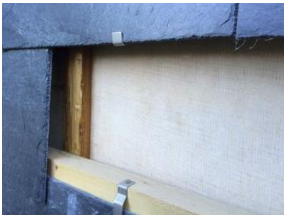
Figure 3: The MgO-board is placed facing the air gap, which is behind the siding boards made of natural slates.
