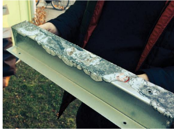
Figure 6: The zink covering of the steel profile is corroded as a result of direct contact with salty sweat or 'tear' drops from the adjacent MgO-board.
