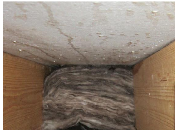
Figure 4: Salty water drops on a vertical MgO-board on the side that faces the insulation filled cavity inside the wall.
