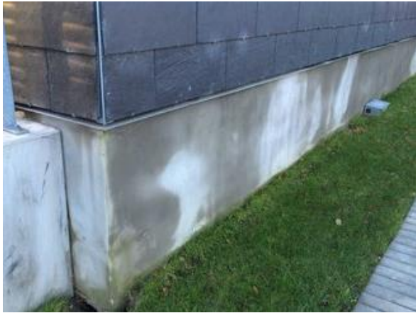
Figure 5: The water drops containing chloride ions run down the vertical MgO-boards and drain out of the wall from behind the wall's siding boards.
